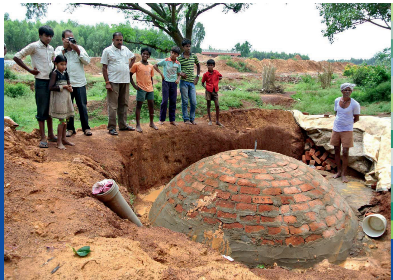
Dome Digester, India – This work © 2018 by BiogasME is licensed under CC BY-SA 4.0.
